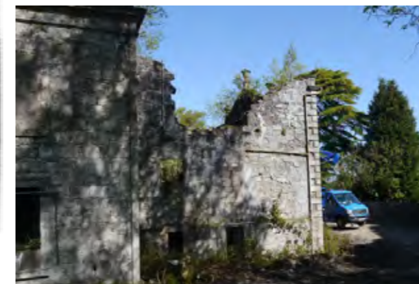
Woodbank House - current ruinous condition
