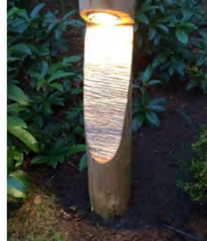
Low level light posts
